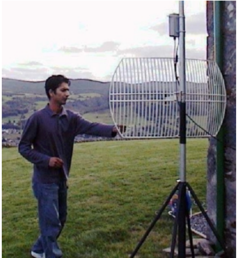
Asif Naser installing the 2.4Ghz TV receiver and retransmitter at the Glassie Bunkhouse above Aberfeldy
